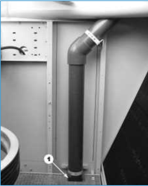
Pump piping plenum section inside
