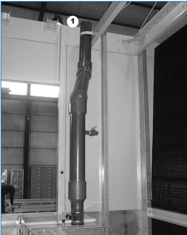
Pump piping lower section
