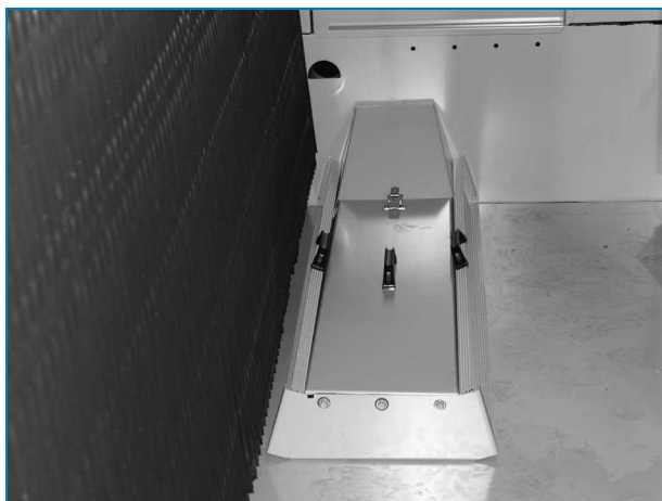
Bazen hladne vode i filter bazena
