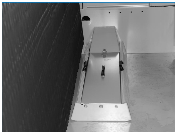
Bazen hladne vode i filter bazena
