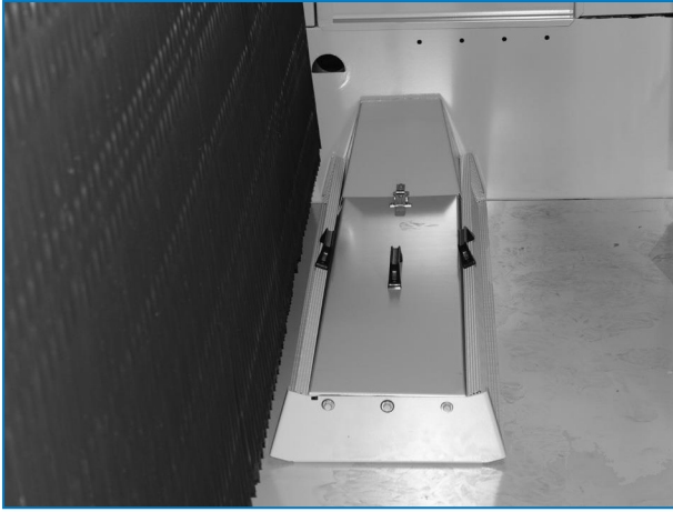
Cold water basin and basin strainer
