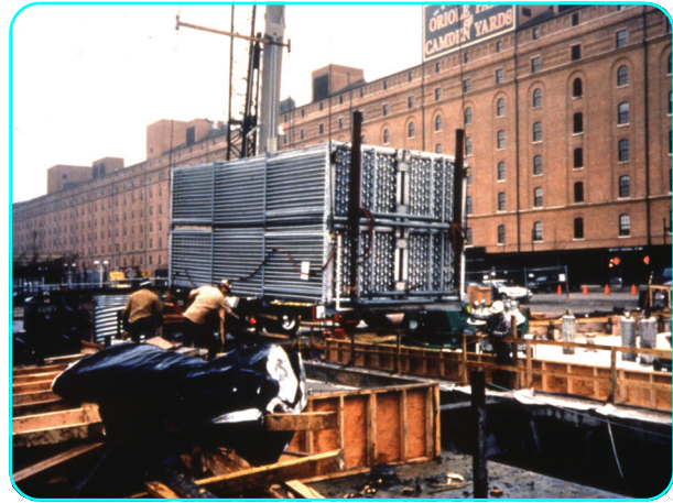
Coils installed in Concrete Tank
