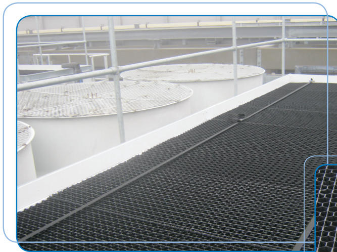
Top Inlet Shields fitted to FXV Closed Circuit Cooling Tower
