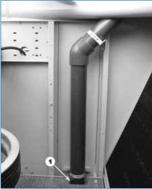
Pump piping plenum section inside
