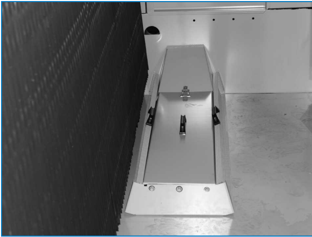
Cold water basin and basin strainer
